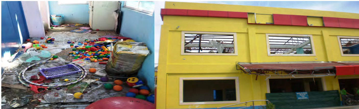
Damaged special education centers
